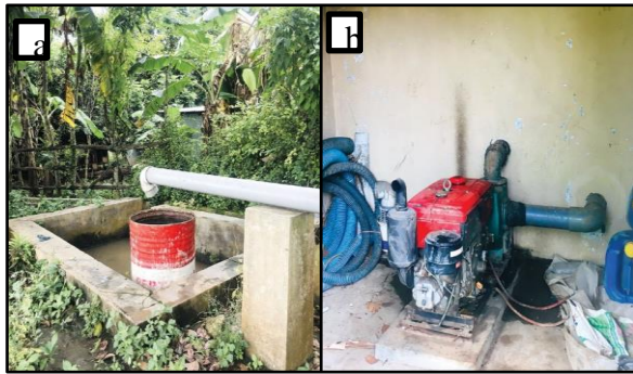
Figure 1. (a) Water Irrigation System Available In The Site; (b) Groundwater Pump Powered By Diesel Generator
