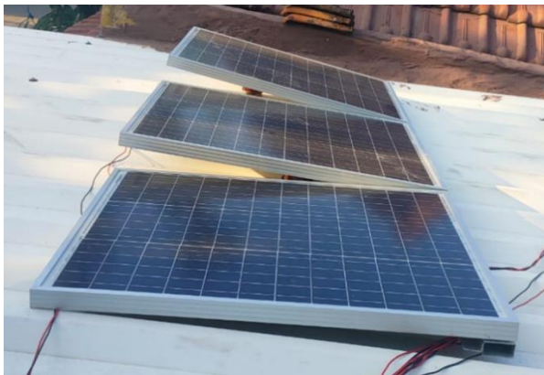
Figure 4. The installation of the tilt angle of the solar panel on the tile on the house's roof
