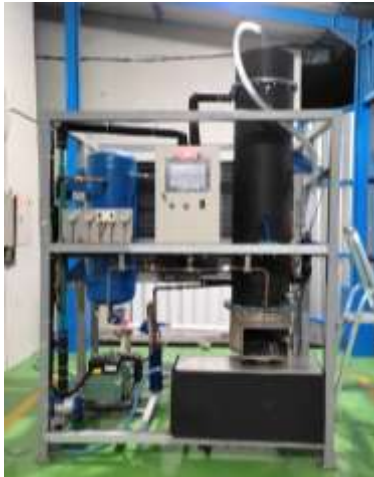
Figure 4. implementation of electrical safety system panels on ice tube machines
