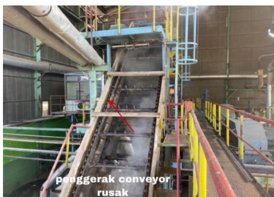
Gambar 6 Fasilitas Dewatering Mill Feed Conveyor
