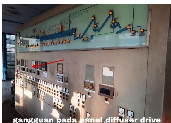
Gambar 7 Panel Diffuser Drive
