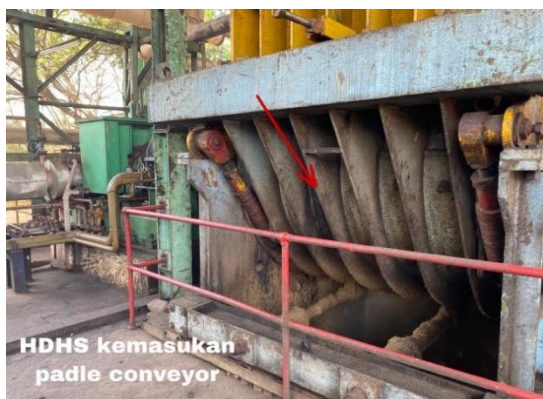
Gambar 10 Fasilitas Heavy Duty Hammer Shredder (HDHS)
